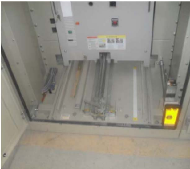
lock on earthing switch
