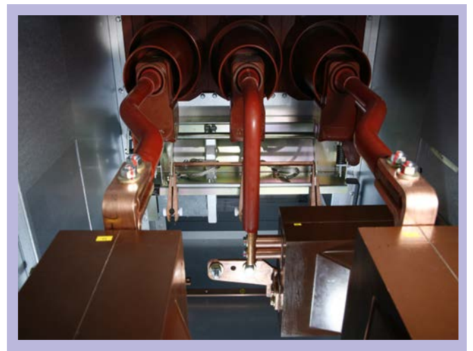
Cable compartment with current transformers
