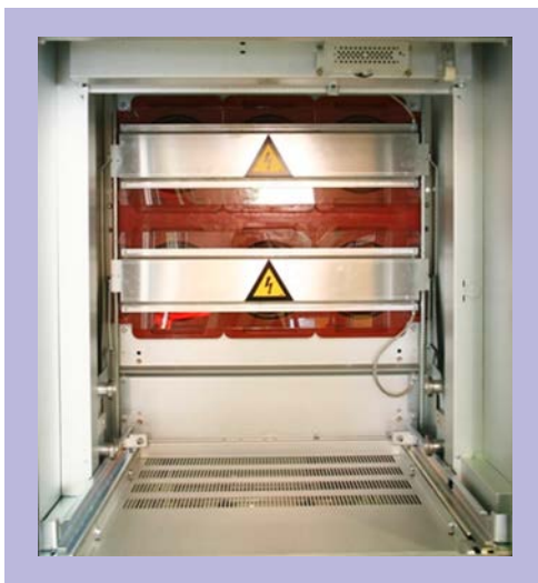
Circuit breaker compartment with shutters
